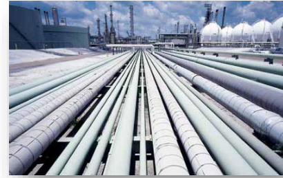
Anti Corrosive Material
