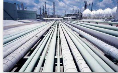
Anti Corrosive Material
